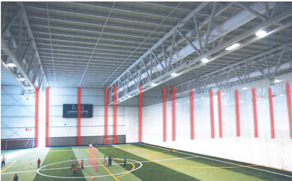
Fig. 18 – Steel columns on the periphery of the building (ABCP infographic on a photograph representing the Victoriaville Complex)
