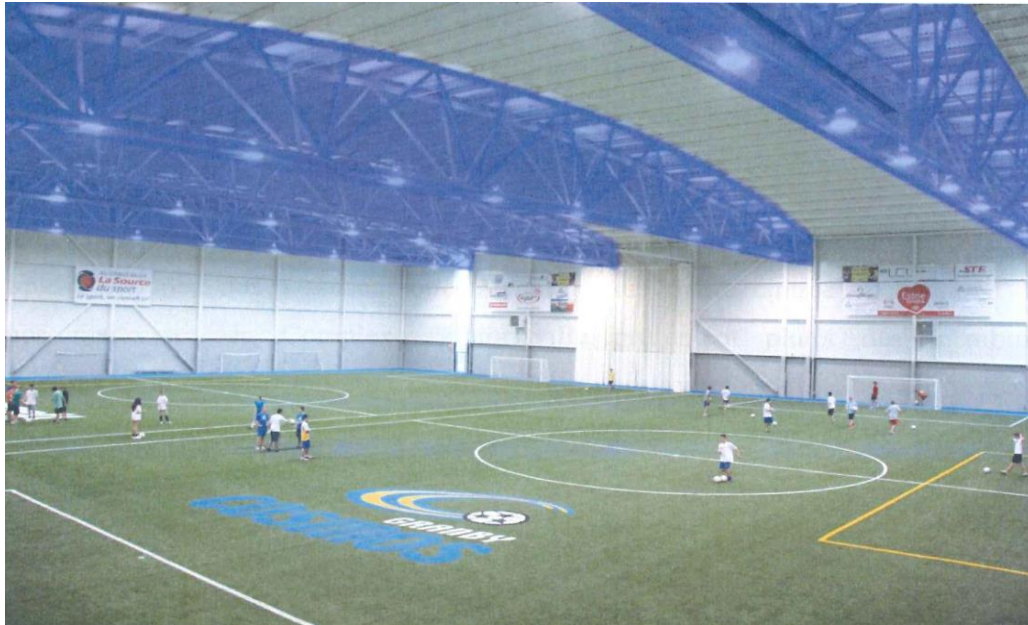
Fig. 19 – Triangular master trusses supporting the cantilever chords (ABCP infographic on a photograph representing the Artopex Complex)
