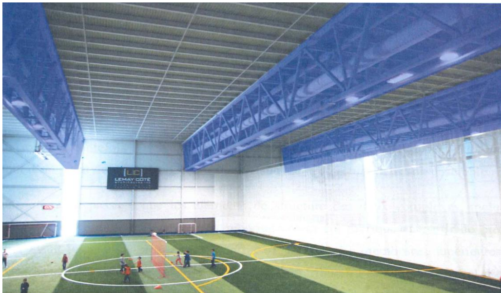
Fig. 20 – Triangular master trusses supporting the cantilever chords (ABCP infographic on a photograph representing the Victoriaville Complex)
